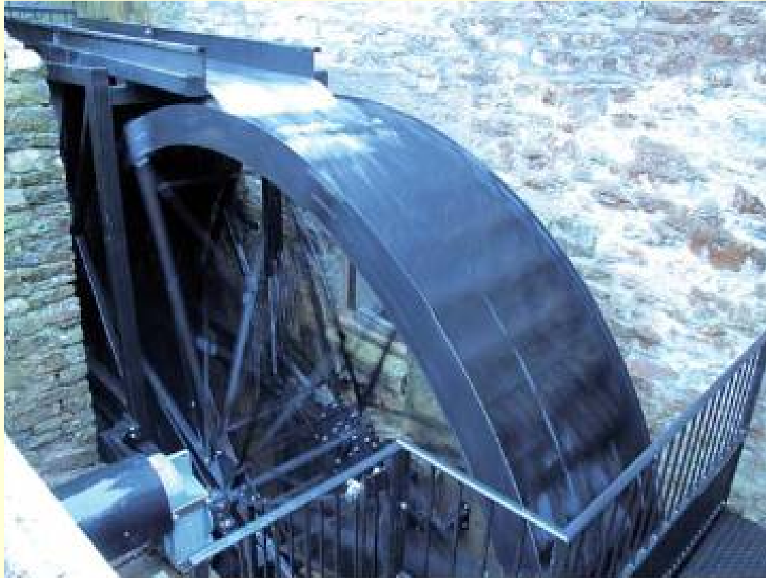
The new wheel at Calver Corn Mill with the very compact generator on the left
